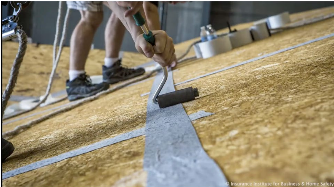
Figure 3. Installing a sealed roof deck system; taping the seams of roof sheathing.
