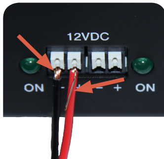
Figure 1.6.1 - Exposed Wire & Poor Connection
