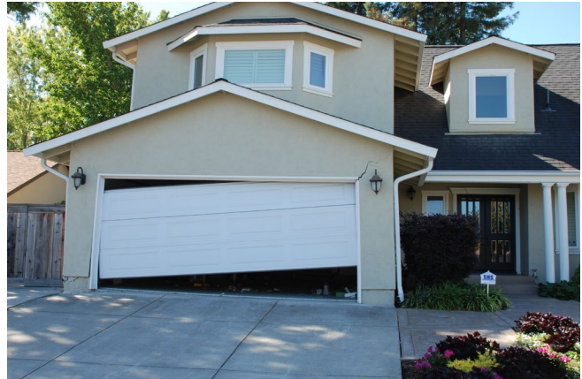
Examples of significant earthquake damage—portions of homes that appear to be leaning or have fallen down.
