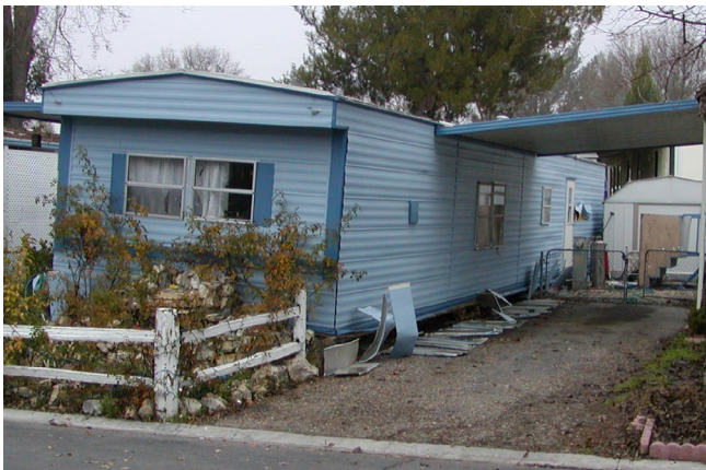
Manufactured home that has fallen off of support piers.
