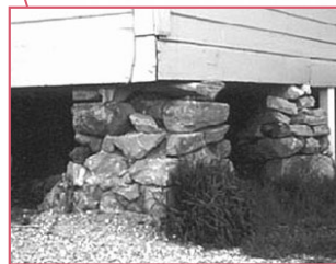
PHOTO COURTESY OF CALIFORNIA SEISMIC SAFETY COMMISSION
