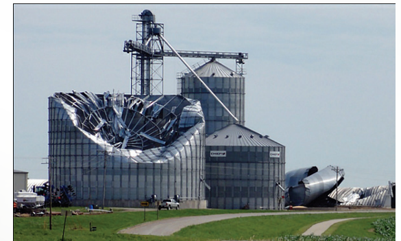
After a tornado, watch out for dangerous debris, such as sharp metal, glass, or downed power lines. Photo: NOAA
