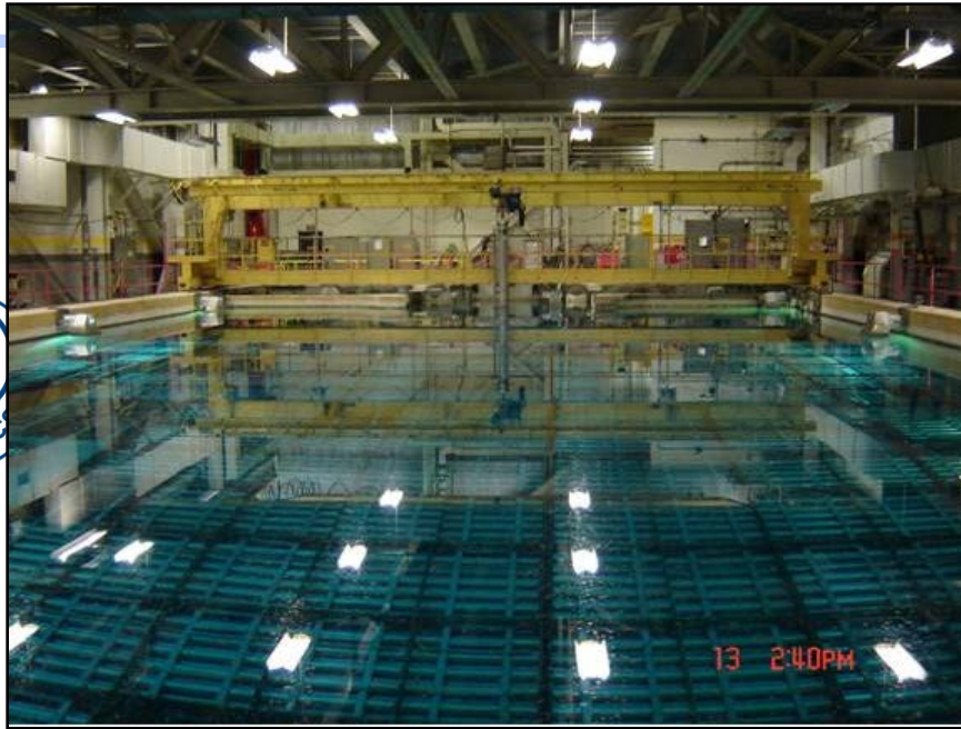
Used nuclear fuel in wet storage within reactor bays
