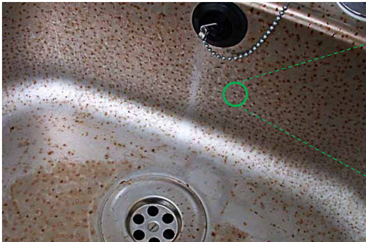
Stainless Steel Pitting
