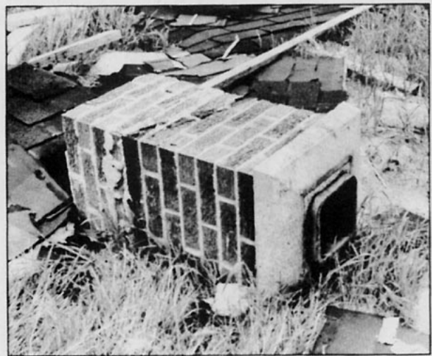
FIG. 26. A close-up view of the 390 lb (180 kg) chimney consisting of 66 bricks, each weighing 5 lb (2.3 kg). (Photo by Fujita and Abbey on 6 August.)
