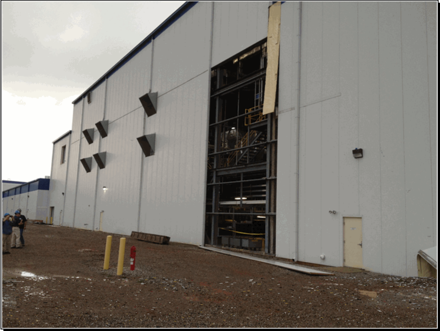
Section of wall blown out at Toray Plant (outside of Decatur) off Hwy 20.
