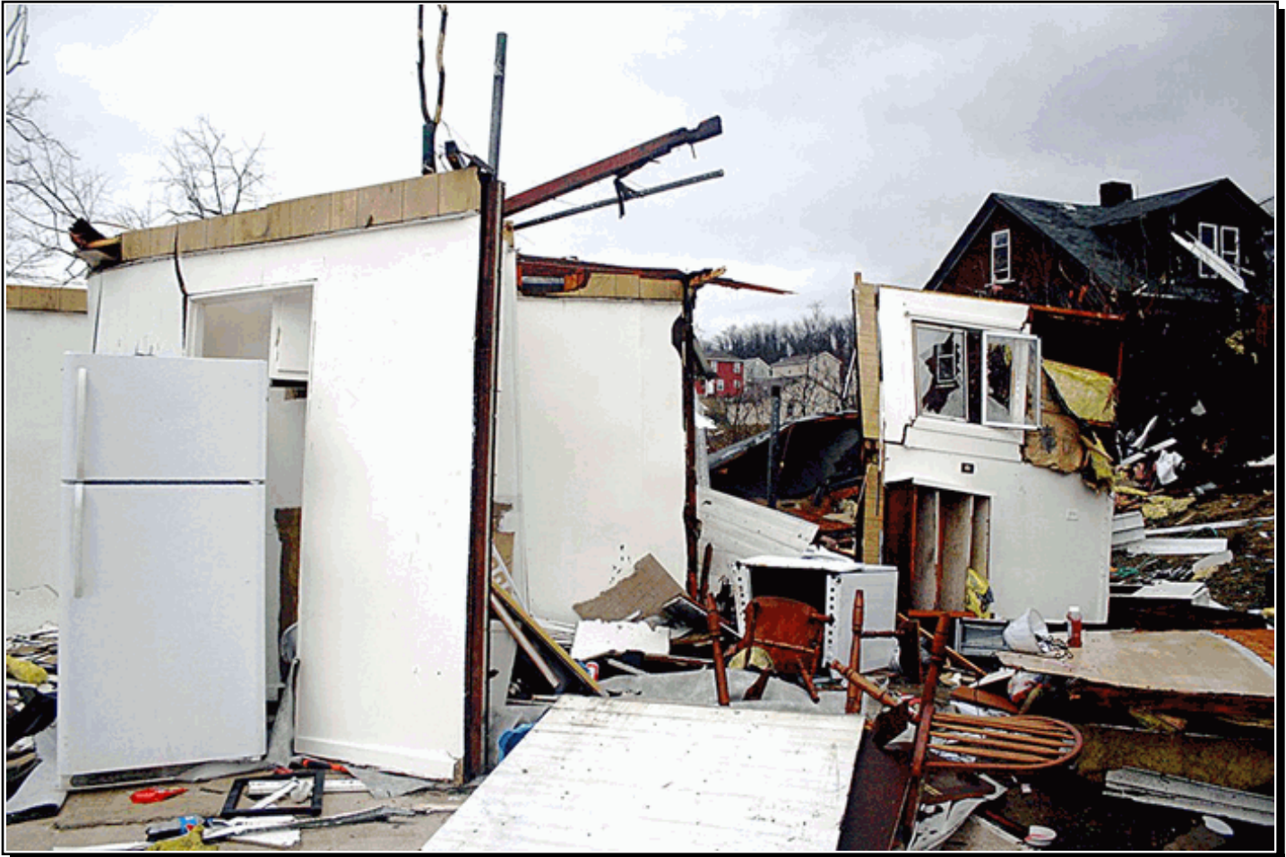
One of the homes that was significantly damaged in Uniontown, Fayette County Pennsylvania on Feb 15th. From the Herald-Standard.
