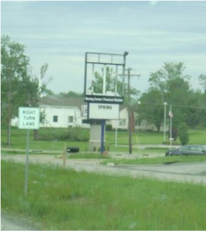
This gas station's canopy over the pumps was levelled...
