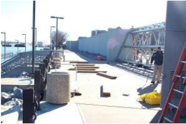
Another photo taken on Friday, Jan. 14 of the floodgate installation in downtown Paducah.
