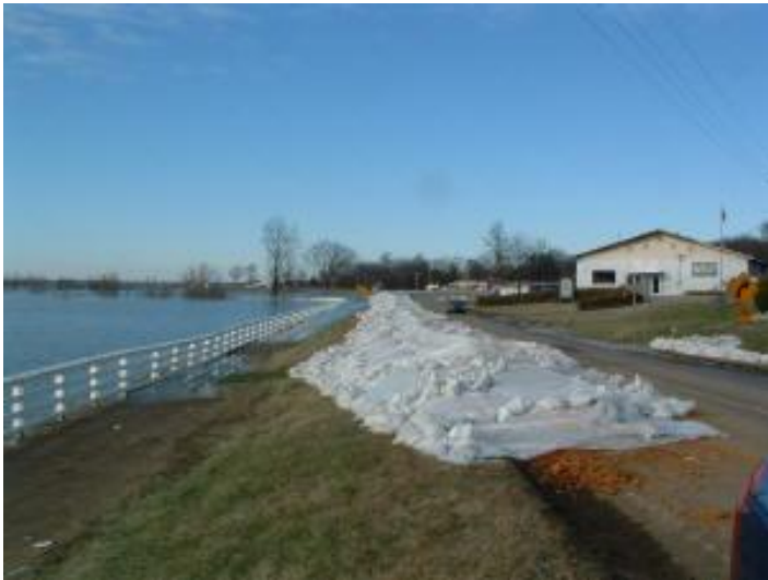
This photo, courtesy of Jeff and Christine Wielgos, shows the makeshift levee constructed on U.S. Highway 60 in Smithland, KY. Smithland is located in Livingston County, about 15 miles upriver from Paducah. With no permanent levee, a makeshift levee is built to protect Smithland during each major river flood. Photo taken looking north on Route 60 from the southern city limits.
