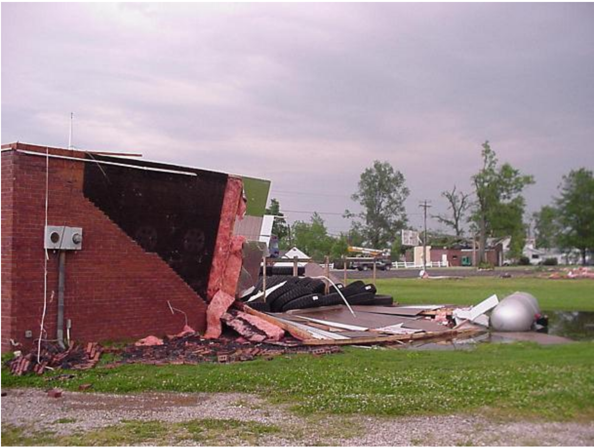
Building with extensive damage
