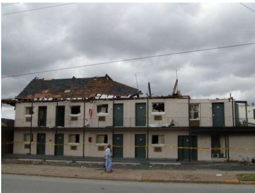
Photo of damage to an Owensboro motel...
