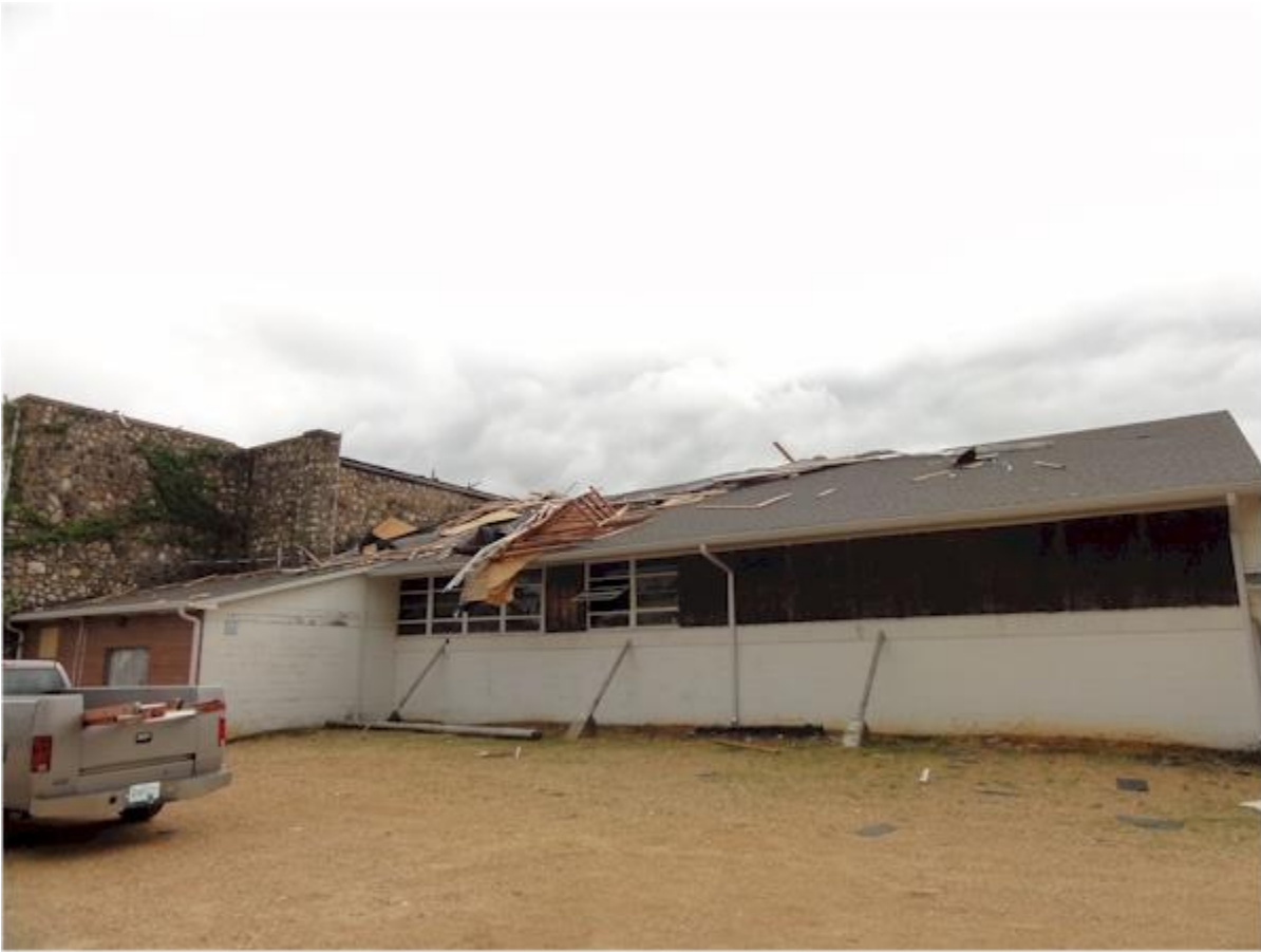
Damage to Grandin School
