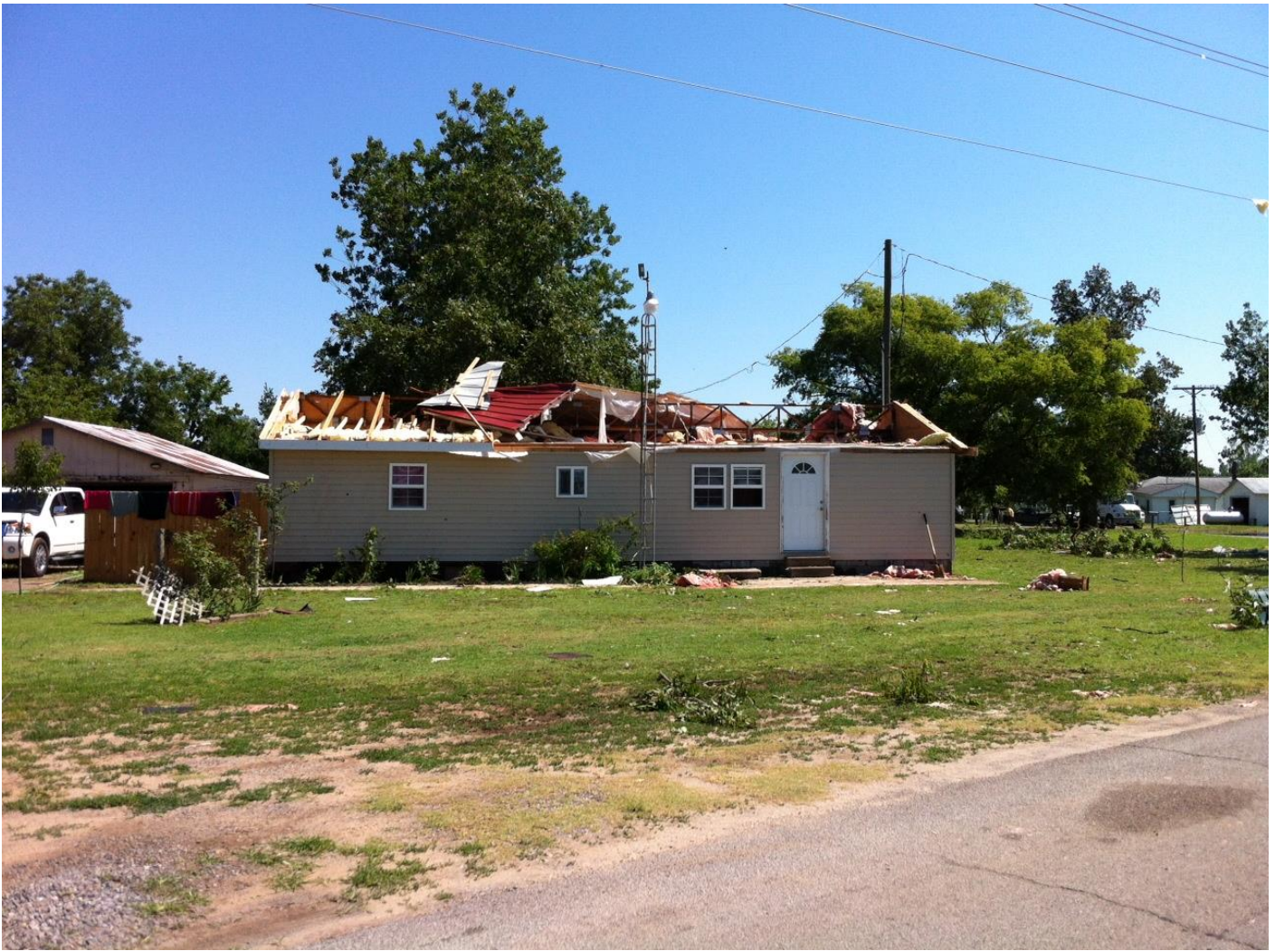
Image of mobile home damaged by downburst in Diehlstadt, MO
