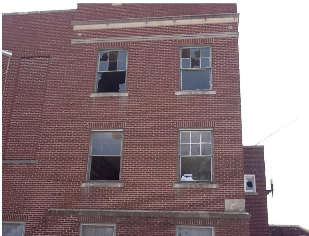
Windows broken in an Oakland City Business
