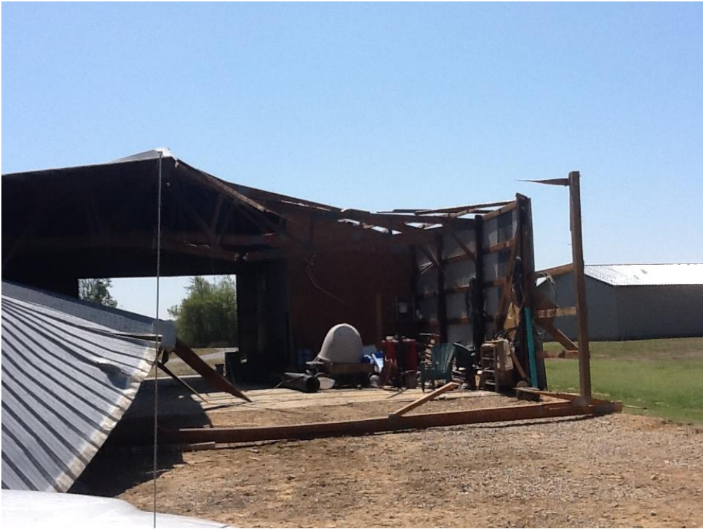
Machine shed destroyed in Oakland City
