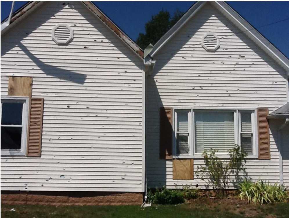
Home damage in Oakland City
