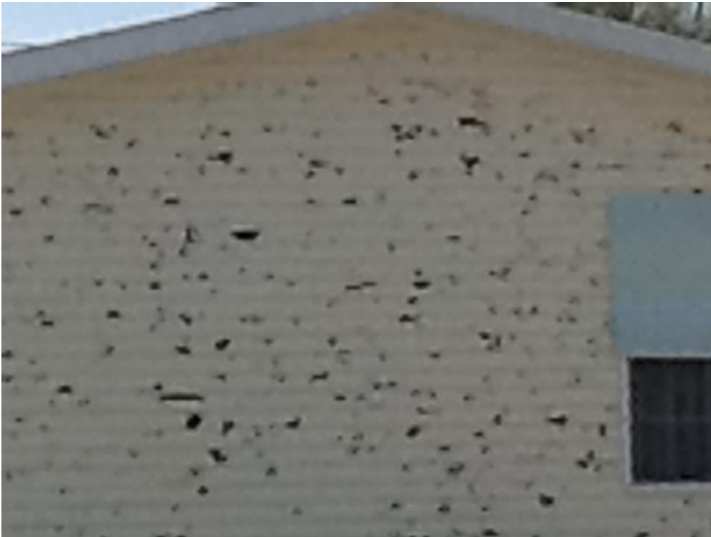
Hail damaged home in Oakland City
