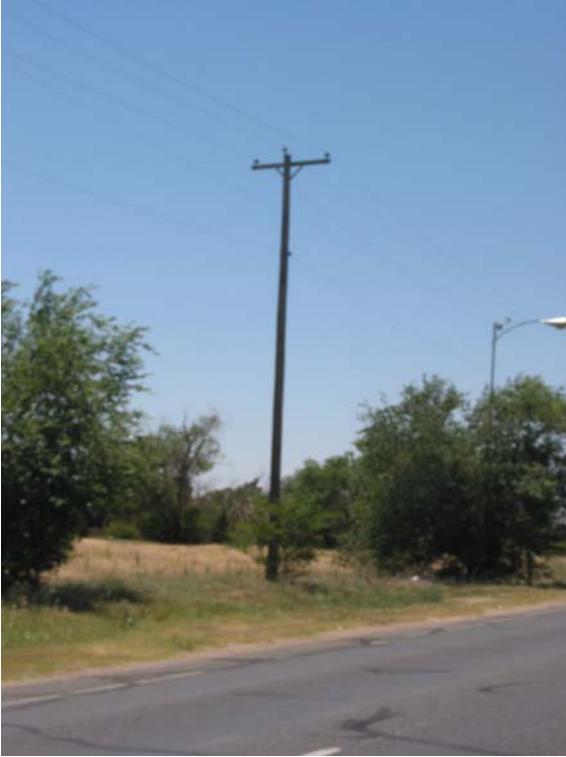
ETL: Single Wood Pole
