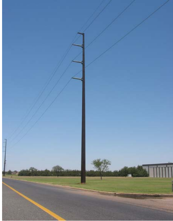
ETL: Single Steel Pole
