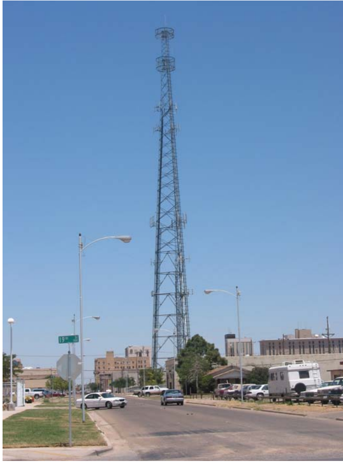
FST: Free-standing Truss Tower
