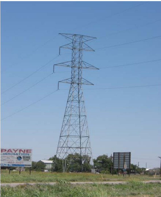
ETL: Metal Truss Tower
