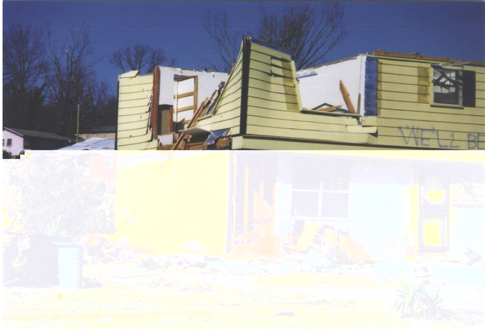
ACT: DOD 4: Uplift or collapse of roof structure leaving most walls standing
