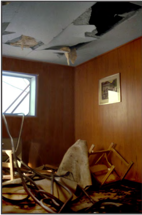
“Stolt Surf” – Junior Officer’s Mess with damaged ceiling, the waves must have been quite violent here (Photography by Karsten Petersen ©)
