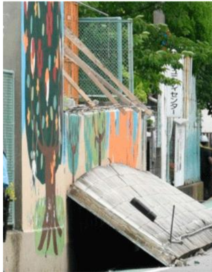
A concrete block wall along a swimming pool, which collapsed during the earthquake (Takatsuki Municipal Juei Elementary School, Osaka Prefecture)
