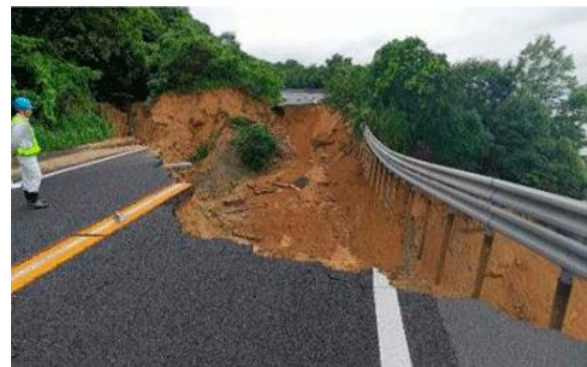
A road cave-in in Mizushiri District, Saka Town, Aki-gun, Hiroshima Prefecture (Hiroshima-Kure Road)
