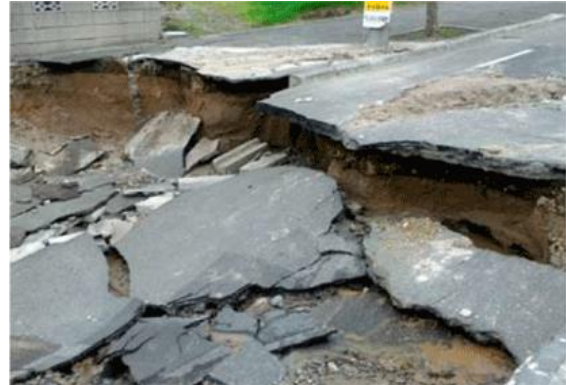
Road failure due to ground subsidence (Hiraoka District, Kiyota-ku)
