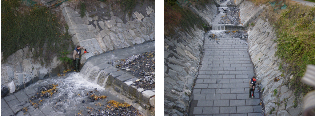
(a) Measuring the cross-section of the main weir (b) Measuring a GRP on the flagstone edges
