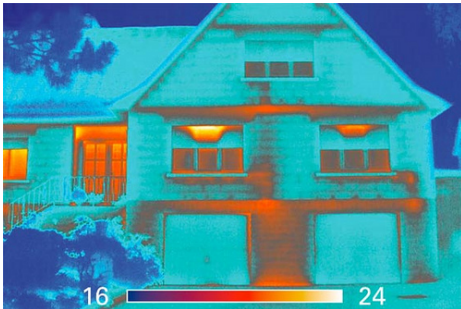
Fig. 9 Thermal image of a building, showing a higher amount of heat loss around windows and doors [149].
